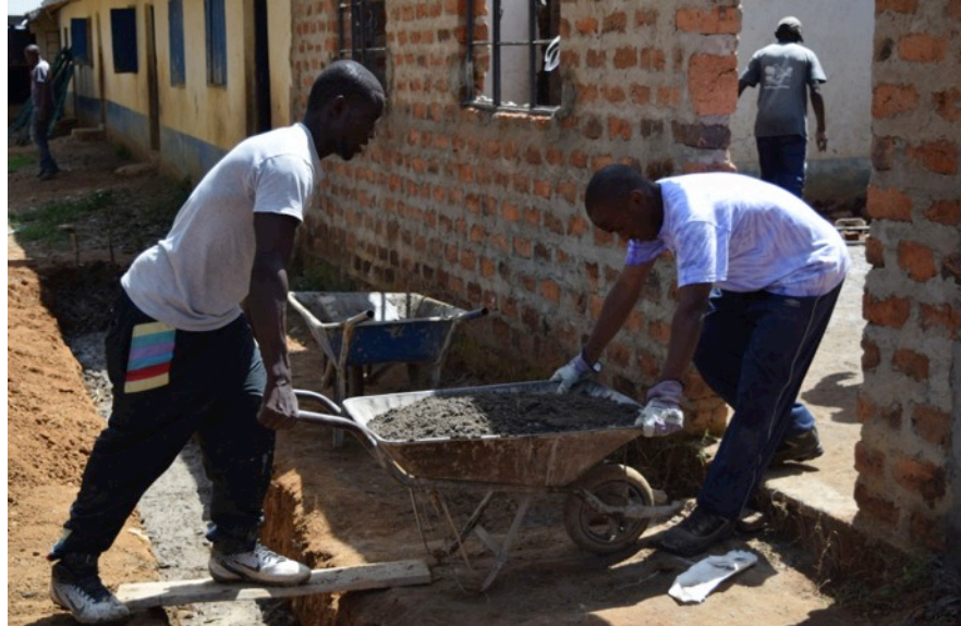
Above: endless wheel barrows, filled with cement and ballast for the walls and floor of the classroom
